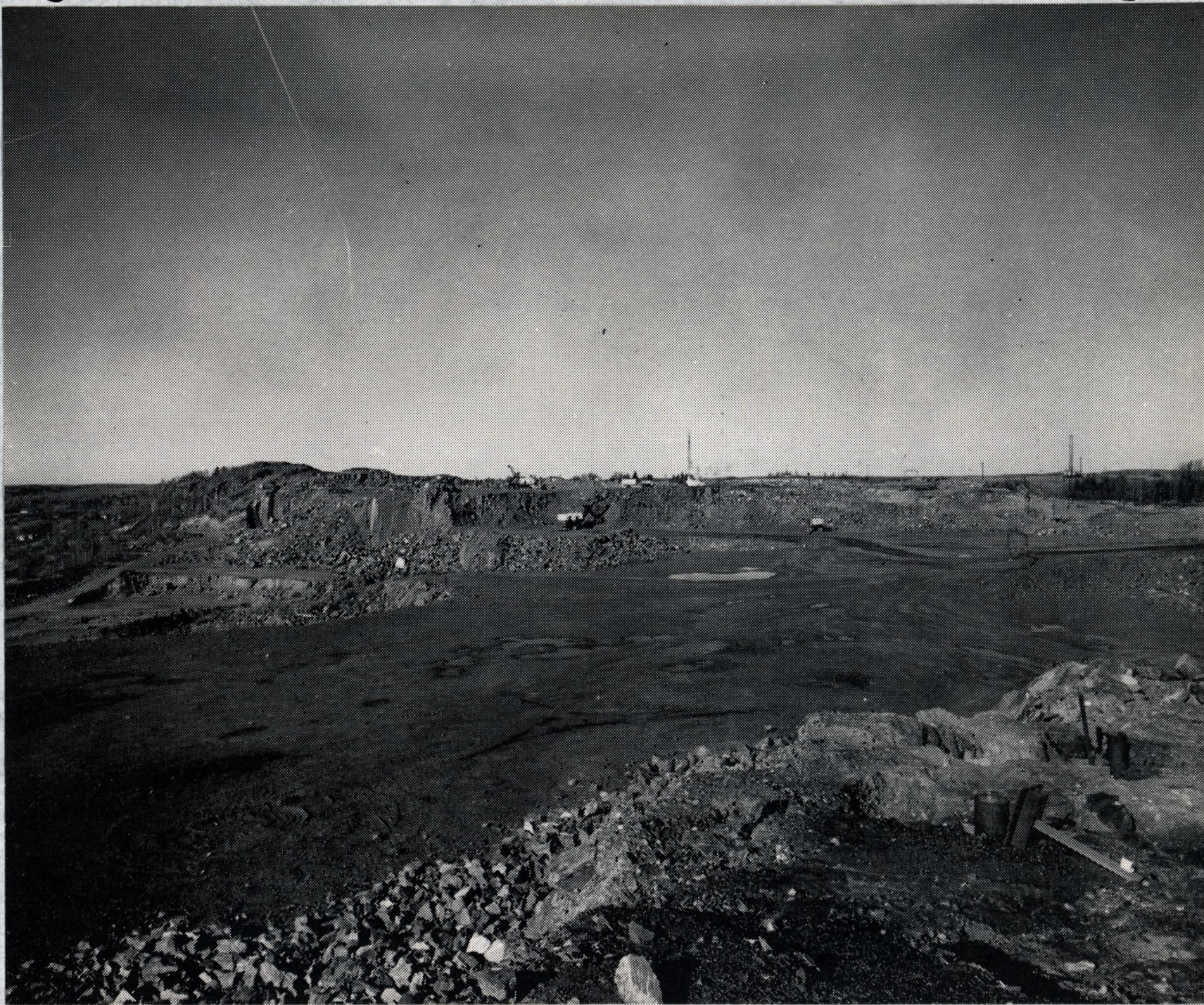
FIG. 2. View of pit looking north. One shovel is shown working on the 1600' bench and the other shovel on the 1640' bench.
