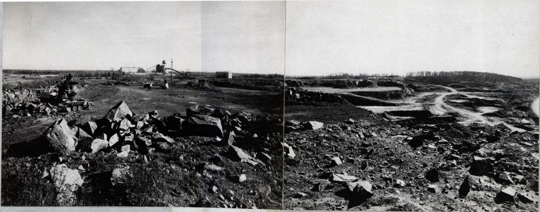
FIG. 3. View looking south, showing shovel at left working on 1640' bench. Road ramping down to 1600' bench is shown just below primary crusher building. Road system on right shows access to proposed 1560' and 1520' benches.
