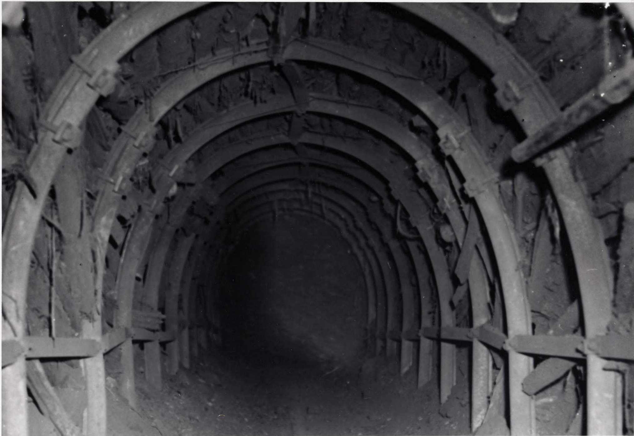
An undercutting drift in a block caving development area utilizing the new yielding arch steel sets as the means of support.
