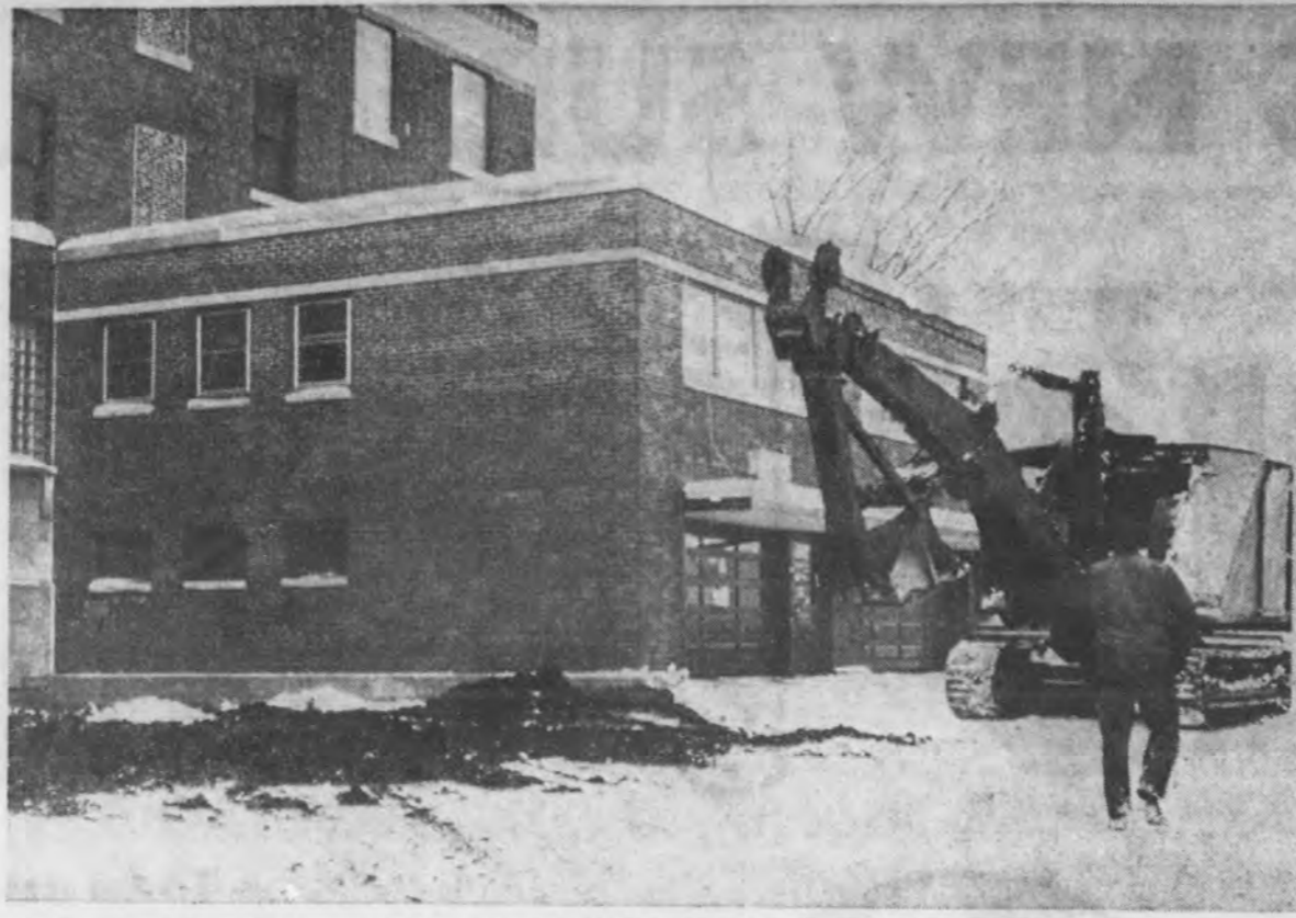
In an area where members of the Bell Memorial Hospital medical staff once parked, the Proksch Construction Co. is now "pile driving" in the initial stages of construction for a $150,000 laboratory addition to the hospital.
