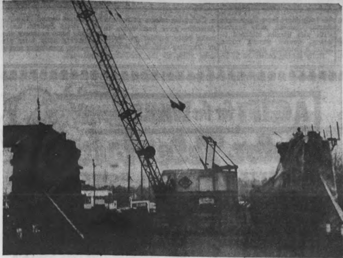
Bridge abutments are being constructed on Third St. (above) and Euclid Ave. to carry tracks for three railroads in rail relocation project in Ishpeming. Another abutment will be erected next year on Second St.—(Mining Journal photo.)
