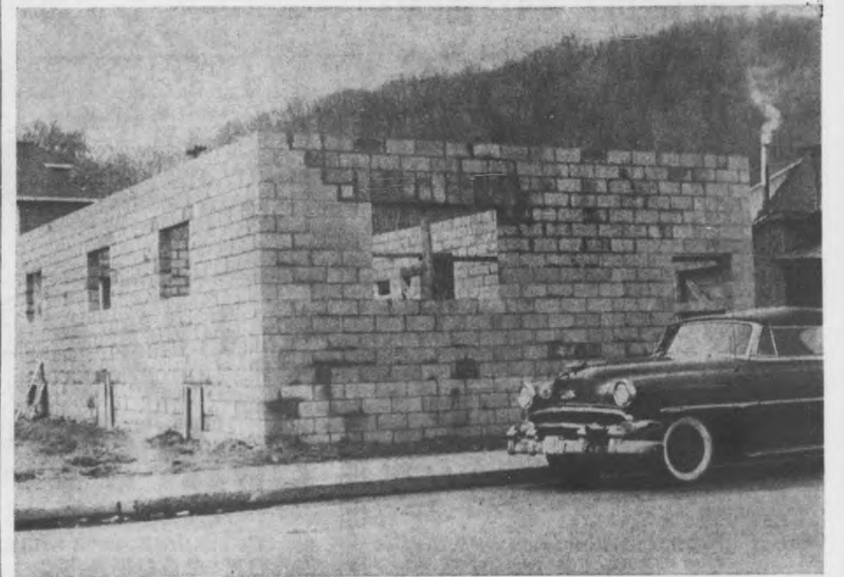
Construction work is progressing on new corner of Superior and Lynn Sts. in Munising. American Legion building being erected at —(Mary Jayne's photos.)
