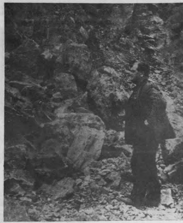
Earl Numinen of Michigamme, project engineer for bypass construction, examines rock that was blasted during work on Marquette route relocation.
