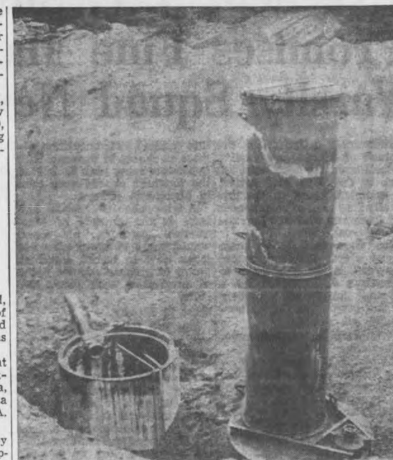
Looking like a rocket pad at a missile base is this classifier digester being constructed in North Ishpeming by the Bahr Construction Co. of Manitowoc, Wis.
