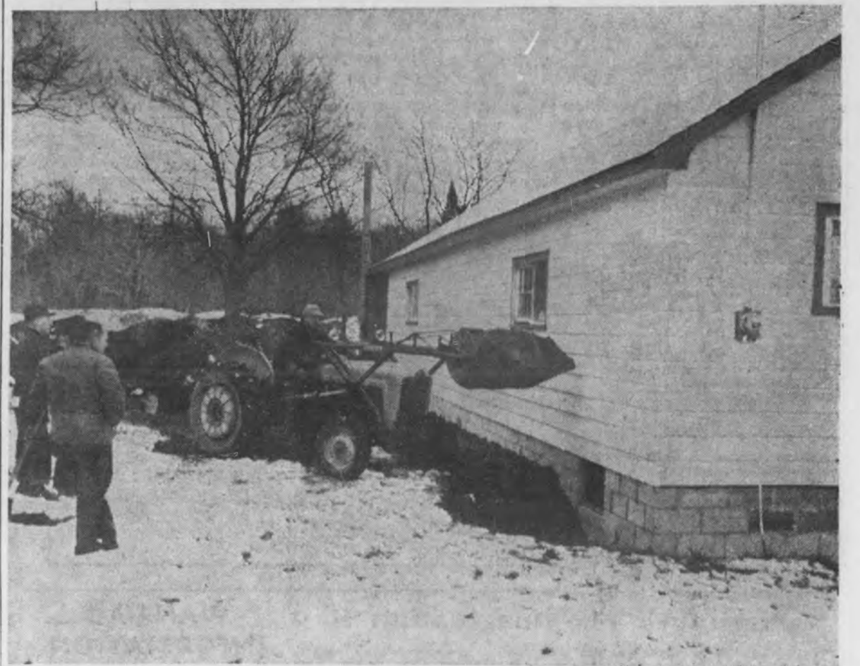
Tractor operator Sonny Cox is shown filling a large container at the new basement at Munising-Alger Conservation Club at Wetmore. The basement, and rest rooms were installed on the first floor which will house a furnace and contain an archery and gun target room, was completed by volunteer members of the organization this fall. The basement, and rest rooms were installed on the first floor which will house a furnace and contain an archery and gun target room, was completed by volunteer members of the organization this fall. The basement, and rest rooms were installed on the first floor which will house a furnace and contain an archery and gun target room, was completed by volunteer members of the organization this fall. (Hallifax photo.)
