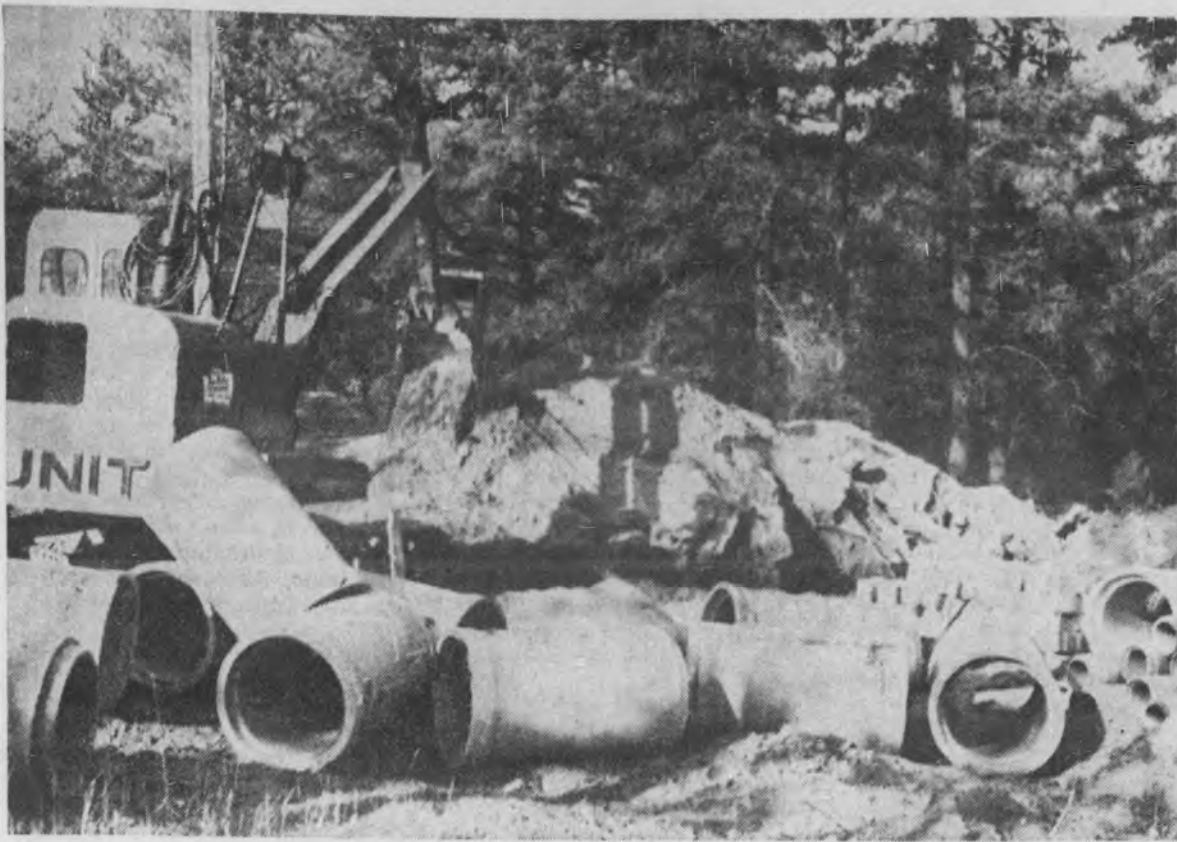
Approximately 400 feet of 24-inch pipe has been laid in Center St. for the storm sewer installation under way north of W. Fair Ave. and west of Lincoln Ave. Don Britton, Marquette, is contractor for the $15,744 project, which calls for the installation of 2,000 feet of storm sewer in Center St., Lynn Ave., Waldo St. and Birch Ave. Work was begun this week on Lynn Ave. Shown here are some of the materials on the job site. The installation project began Nov. 1, and, weather permitting, will be completed by the end of the month.—(Mining Journal photo.)
