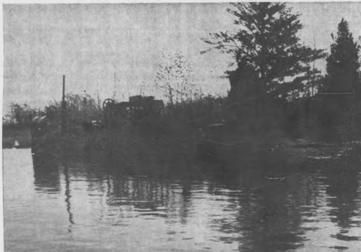
Shown above is large dredge used to transfer up to 300 cubic yards of sand fill a day from lagoon area to swamps to construct a roadbed and to dredge out lagoon for a harbor at the park. Road to be built over swamp will provide access to beach where picnic tables will be located and campsites developed. (Mining Journal photos.)
