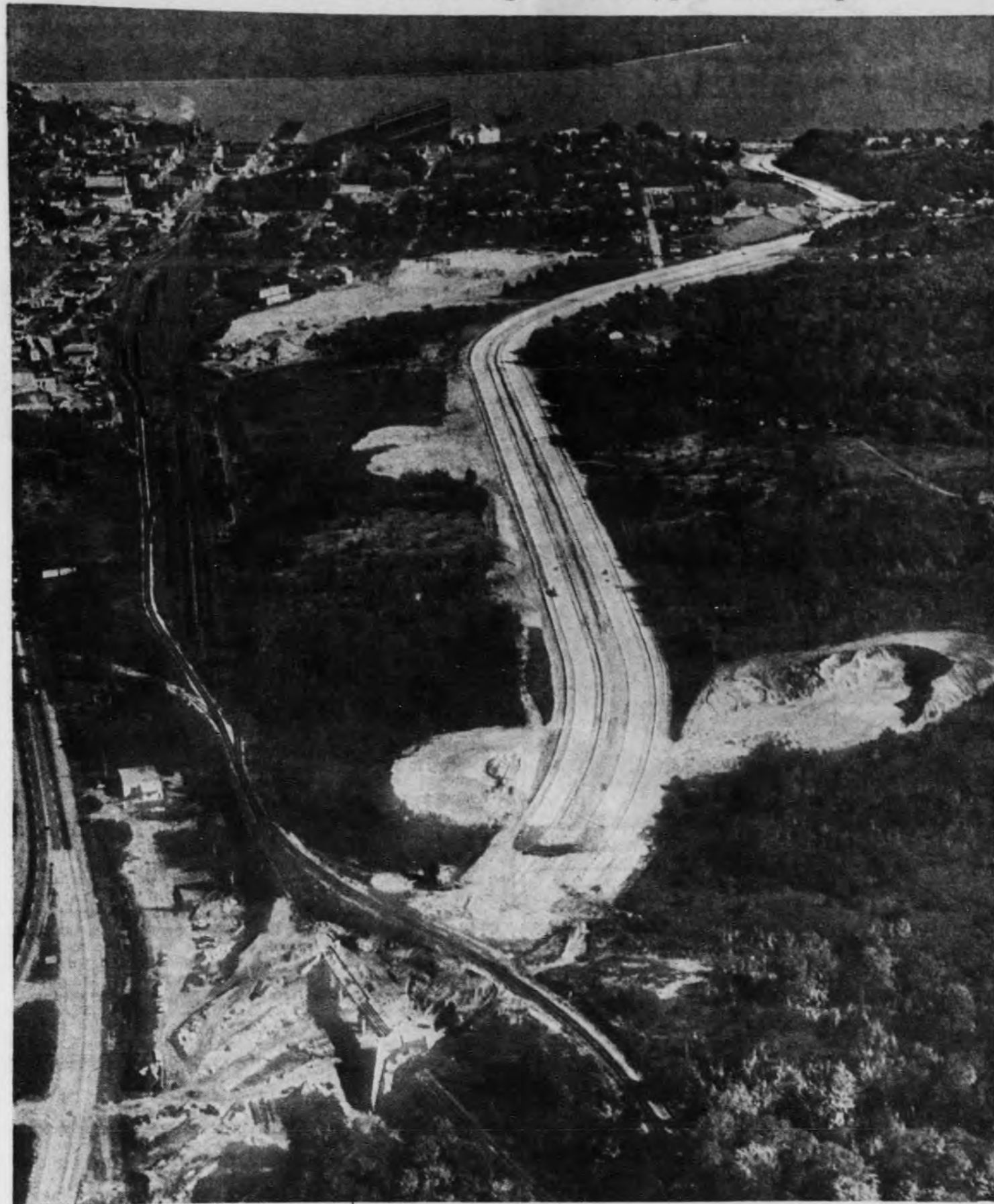
This aerial view, taken by Mining Journal Photographer Bill Williams, shows the route of and progress being made on the U. S. 41 and M-28 route relocation in Marquette. The foreground shows the work at the Soo Line Railroad Co. overpass, with the bypass connecting with existing U. S. 41 in the Brewery Location (lower left of picture). Holy Family Home can be seen
