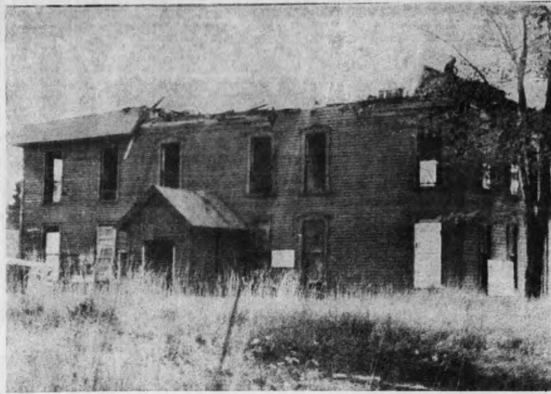
Marquette Public Schools' old special education building on E. Ridge St. is being razed by Robert Gerardi of G and L Home Builders of Negaunee, who purchased the eight-lot Howard-Froebel property this spring. The residence was purchased by the public schools in 1900 for future expansion of the Howard - Froebel School. The building was used for special education classes until the school was vacated in the fall of 1960 and was then used for storage space until this spring.—(Mining Journal photo).
