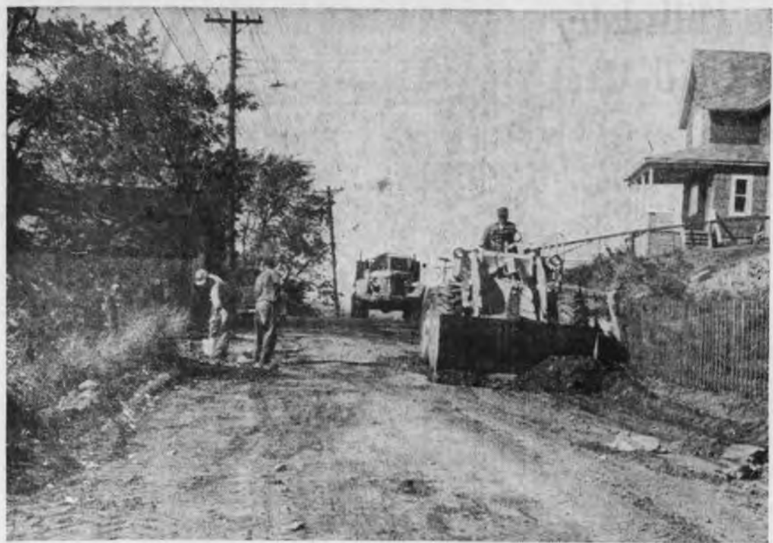
L. W. Brumm Construction Co. crews are laying 31,000 feet of pipe in 118 working days, less than half the time called for in original contract.—(Mining Journal photo).
