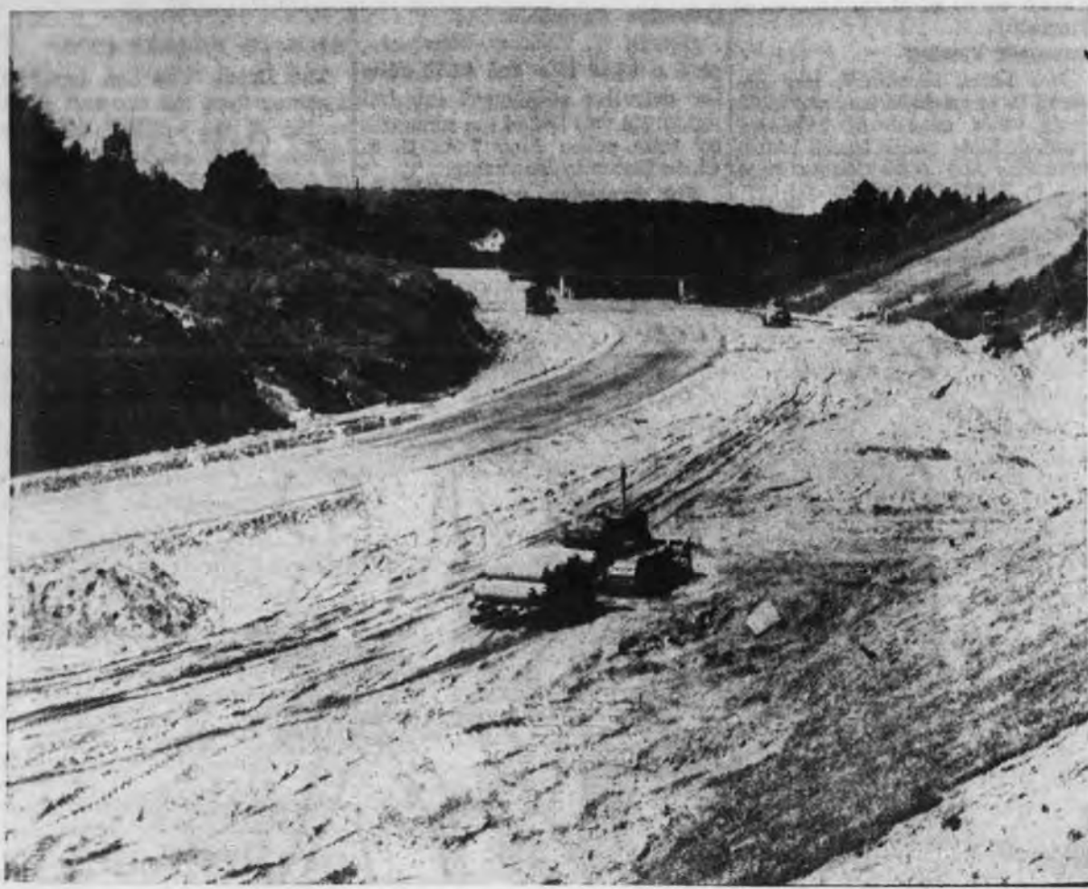
This view of the U.S. 41 and M-28 route relocation in Marquette was taken last week just before the paving work was started. Picture was taken from the Champion St. crossing, showing the Altamont St. overpassing in the background. Much of the paving in connection with the 1.7-mile
