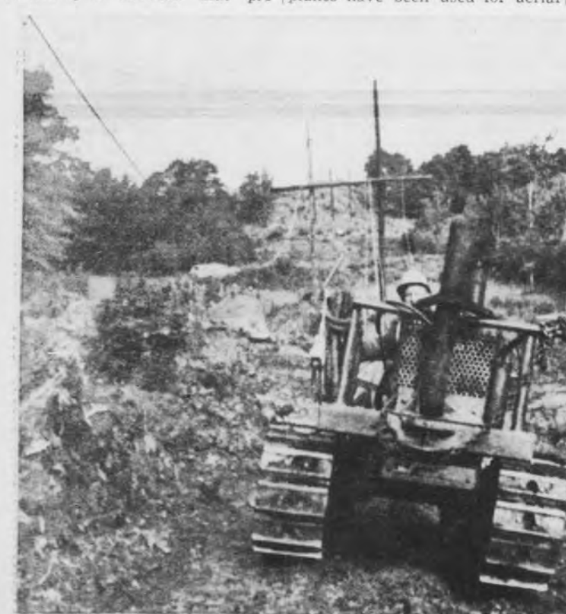
Following decision to abandon aerial installation attempt Thursday, tractor driven by Elmer Palmer began pulling nearly-inch-thick cables across rough terrain that runs from Cedar Lake eastward behind Suicide Hill. Three cables, each weighing 833 pounds per 1,000 feet, are being placed on spans already set up on 3 1/2-mile transmission route. — (Mining Journal photos.)
