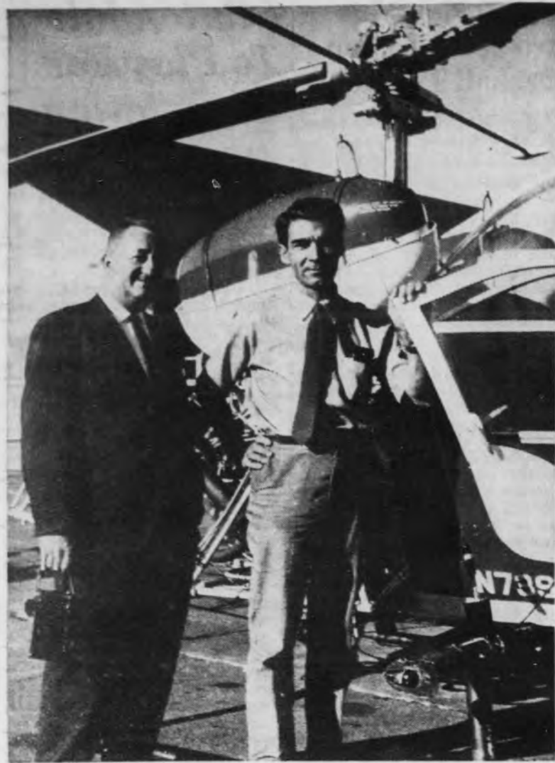
Frank Wheatlake (left), president of power line building firm, and Bill Loftus, pilot, are shown at Marquette County Airport beside helicopter used in attempt to install cable from Upper Peninsula Power Co.'s Cedar Lake substation to Empire Mine.
