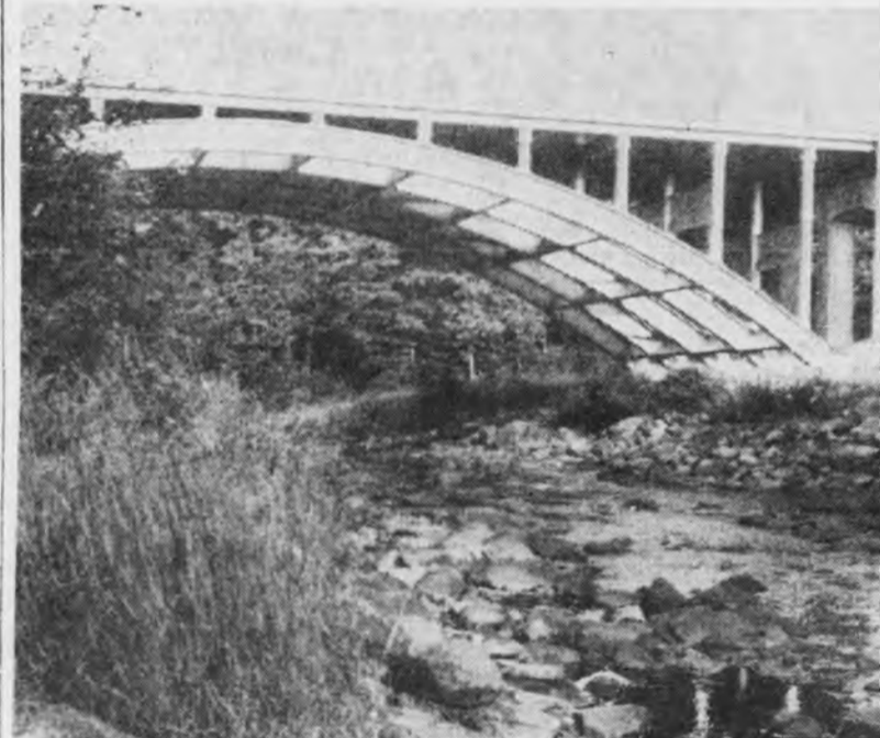
Effect of prolonged dry spell in Baraga County area is dramatically depicted in this picture of the Sturgeon River under bridge over U.S. 41 near Alberta. Normally a broad stream, the Sturgeon has been reduced to a trickle and its famed Sturgeon (Baceo) Falls is a mere shadow of its normal spectacular self.
