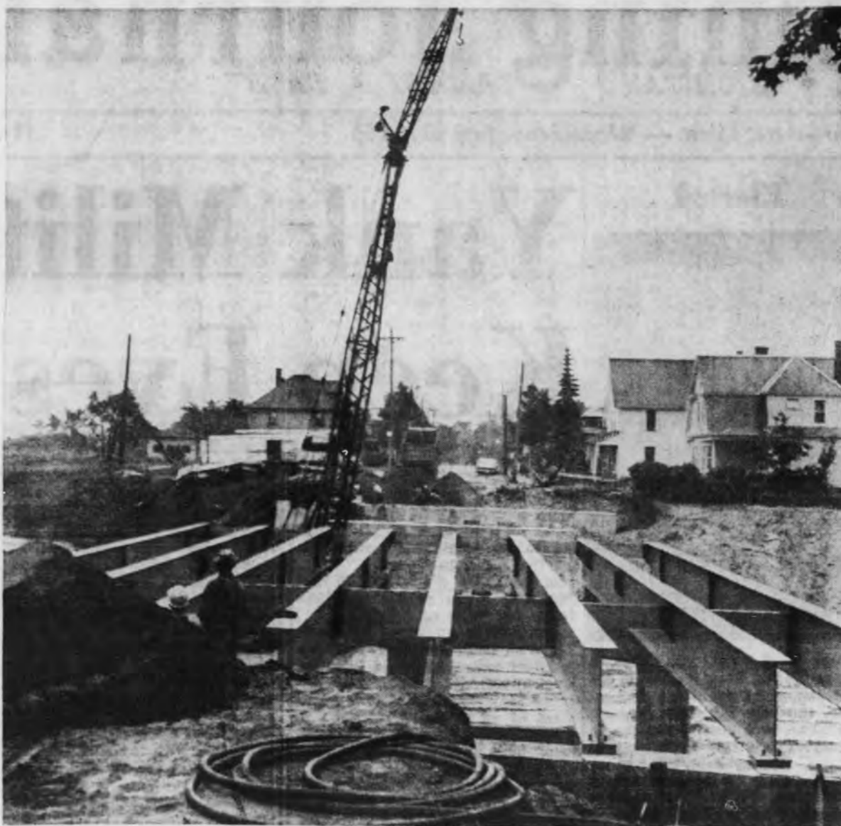
Construction of the Champion St. overpass on the U.S. 41 and M-28 route relocation in Marquette has been started. Photo shows some of the long steel beams being put into place by use of a large crane. Work is being done by the Bacco Construction Co., Iron Mountain, which has the general construction contract, totaling $1,078,446.80. Another overpass will be erected at the Altamont St. intersection. There will be only one other cross-over on the bypass, at grade, at Grove St. Another overpass, for the Soo Line Railroad Co. tracks at the west city limits, is being done by another contractor. Work on the bypass began last fall and is expected to be completed by next summer. It will extend 1.7 miles, from the Brewery Location to Palms St., and will be four lanes of divided highway. — (Mining Journal photo.)
