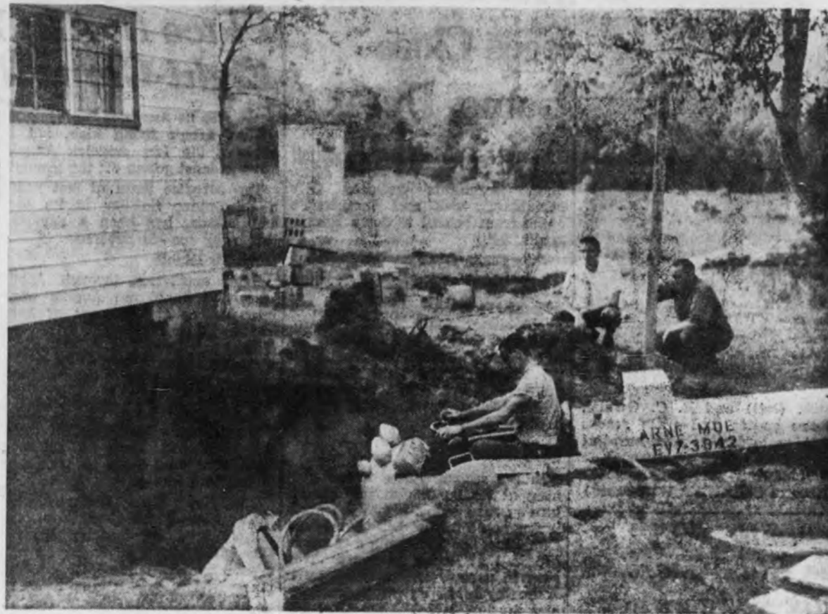
Work has begun on installing a full basement beneath the Munising-Alger Conservation Club building east of Wetmore on M-28. When completed, the new facility will include a new furnace for the building, a range for the junior rifle club, an archery range and toilet facilities. Pictured are volunteer workers engaged in digging operation for new basement. Much of the labor will be donated by members of the organization. (Photo by Dick Hallifax.)
