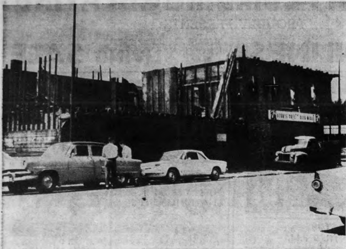
One of Ishpeming's oldest buildings is being torn down in another effort by Ishpeming businessmen to improve the appearance of the business district. Pictured is the Senate Cafe owned by the Nardi brothers of Ishpeming. Plans for the 70 x 100 foot lot are not completed, but once the lot is cleaned of the debris, it will be used for parking. The building is located on the corner of First St. and Cleveland Ave. (Mining Journal photo).
