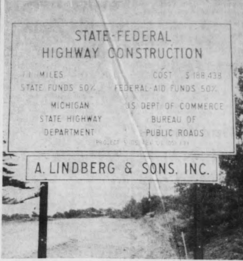
Sign discloses pertinent information concerning road project west of Ishpeming, including cost of 1.1-mile job — $188,438.
