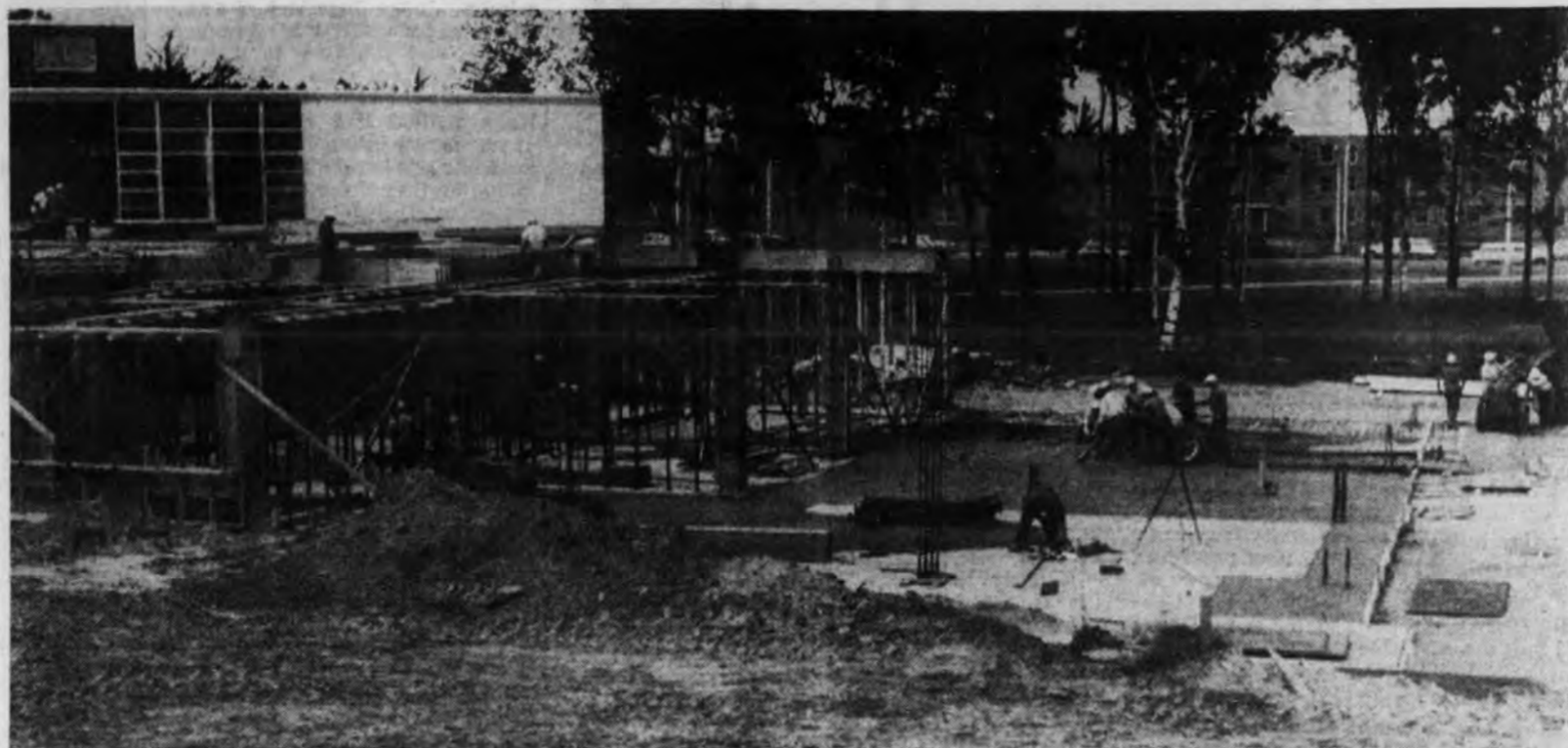
Work is proceeding satisfactorily on the addition to the University Center at Northern Michigan University. The steel framework for the extension is shown here, extending eastward from the existing (background, left) center. In background (right) is the college's Spooner Residence Hall. Miller, Davis and MacDonald of Kalamazoo
