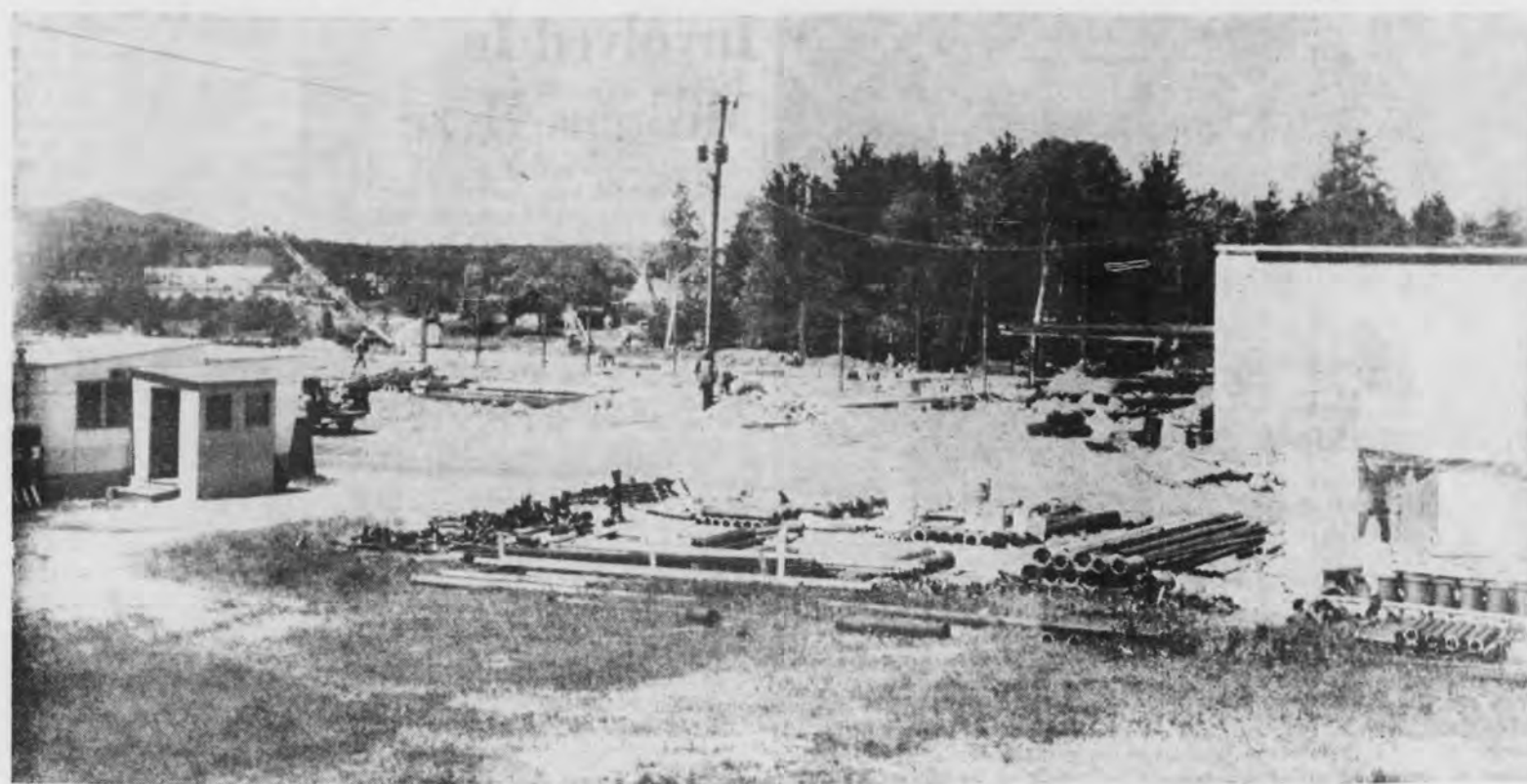
Construction work on the new Practical and Fine Arts Building at Northern Michigan University has projected westward, across what formerly was N. Eighth St., north of W. Fair Ave. Photo shows portion of completed structure (at right) and foundation work, sewer and water line extensions (following utility wire route) to the west. Work on the $2,650,000 building began last September by the Herman Gund-
