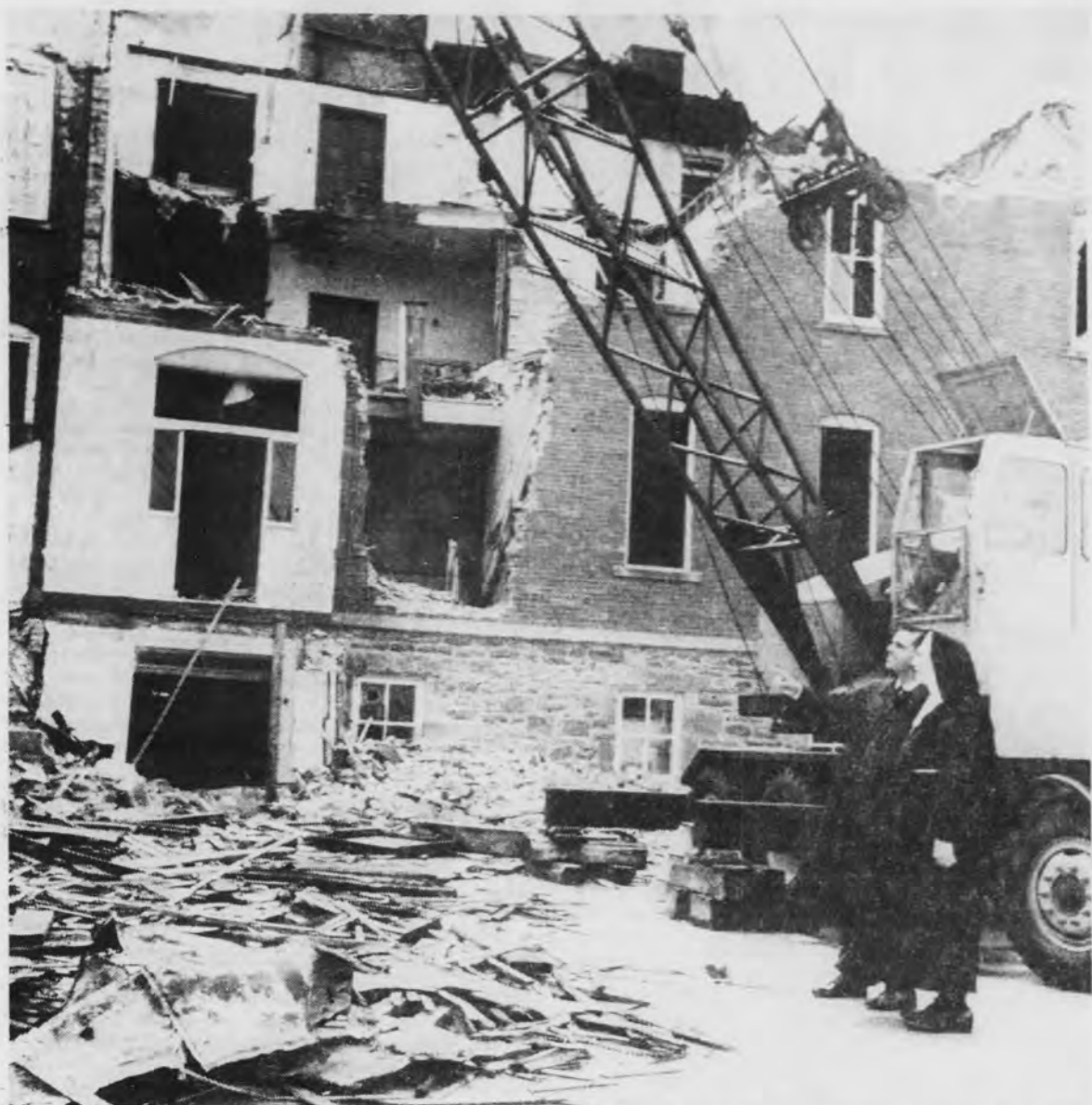
Sister M. Bonaventura, administrator of St. Mary's Hospital, and George P. Mancuso, assistant administrator, inspect the demolition work at Old St. Mary's Hospital building. The building, located immediately east of the new building, is being razed by the Madison (Wis.) Wrecking Co. The building will be completely torn down by June 1. (Mining Journal photo.)
