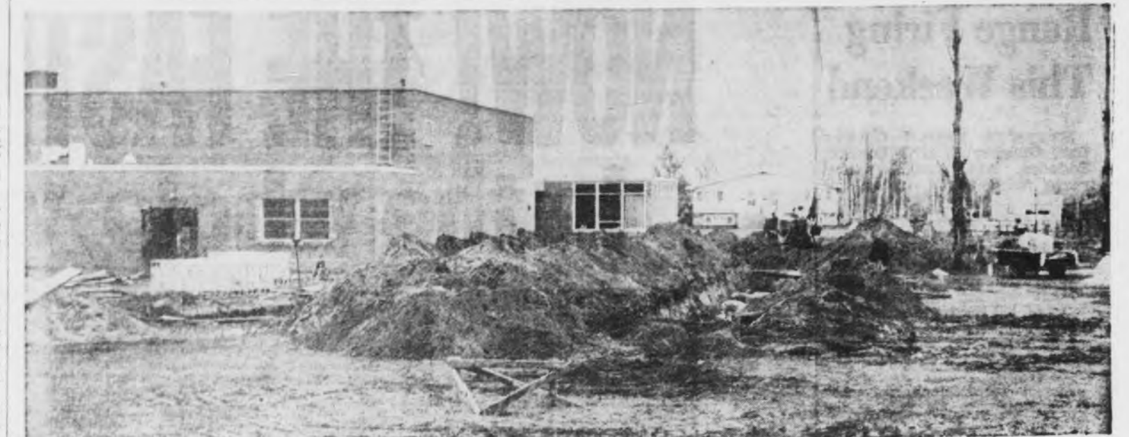
Construction work has been started on the new six-classroom addition to the Sandy Knoll School. General contractor for the work is Sappala Construction Co. Inc., Marquette. Sappala's contract is in the amount of $77,770, with the overall project, scheduled to be completed by Sept. 1 this year, costing around $116,000. This view shows workers preparing the foundation for the new addition, which will extend southwestward from the present building, toward N. Seventh and W. Ridge Sts.—(Mining Journal photo).
