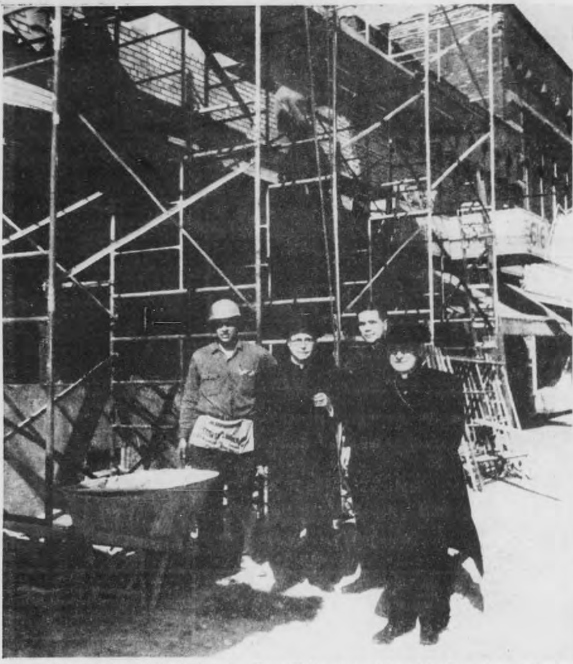
Inspected recently was the Bishop Noa Home for Senior Citizens, under construction in Escanaba. On the inspection tour were the Most Rev. Thomas L. Noa, D.D., bishop of the Catholic Diocese of Marquette, at left; the Rt. Rev. Msgr. Martin B. Melican (second from left), Escanaba, and the Rev. Dominic Zadra, Marquette, chancery officer, secretary to the bishop. Construction worker is Herman Menze of Menze Construction Co., Inc., of Marquette.
