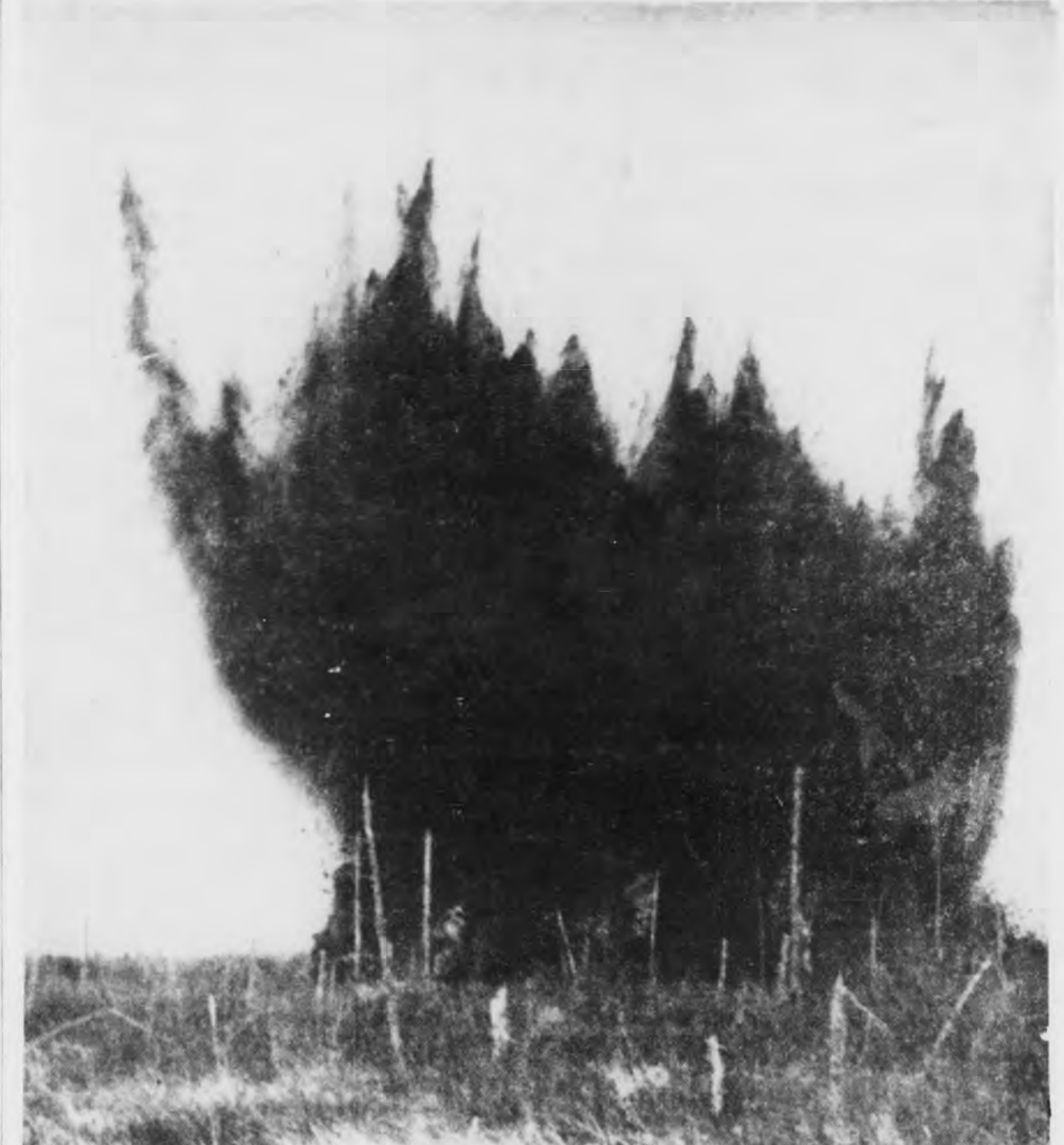
Skyward go tons of Tawas peat, much of it frozen to a depth of more than a foot, as U. S. Forest Service blasters open a ditch in the St. Jacques Marsh on the west branch of the Ogontz River in the Hiawatha National Forest to create more "edge" for a duck factory.
