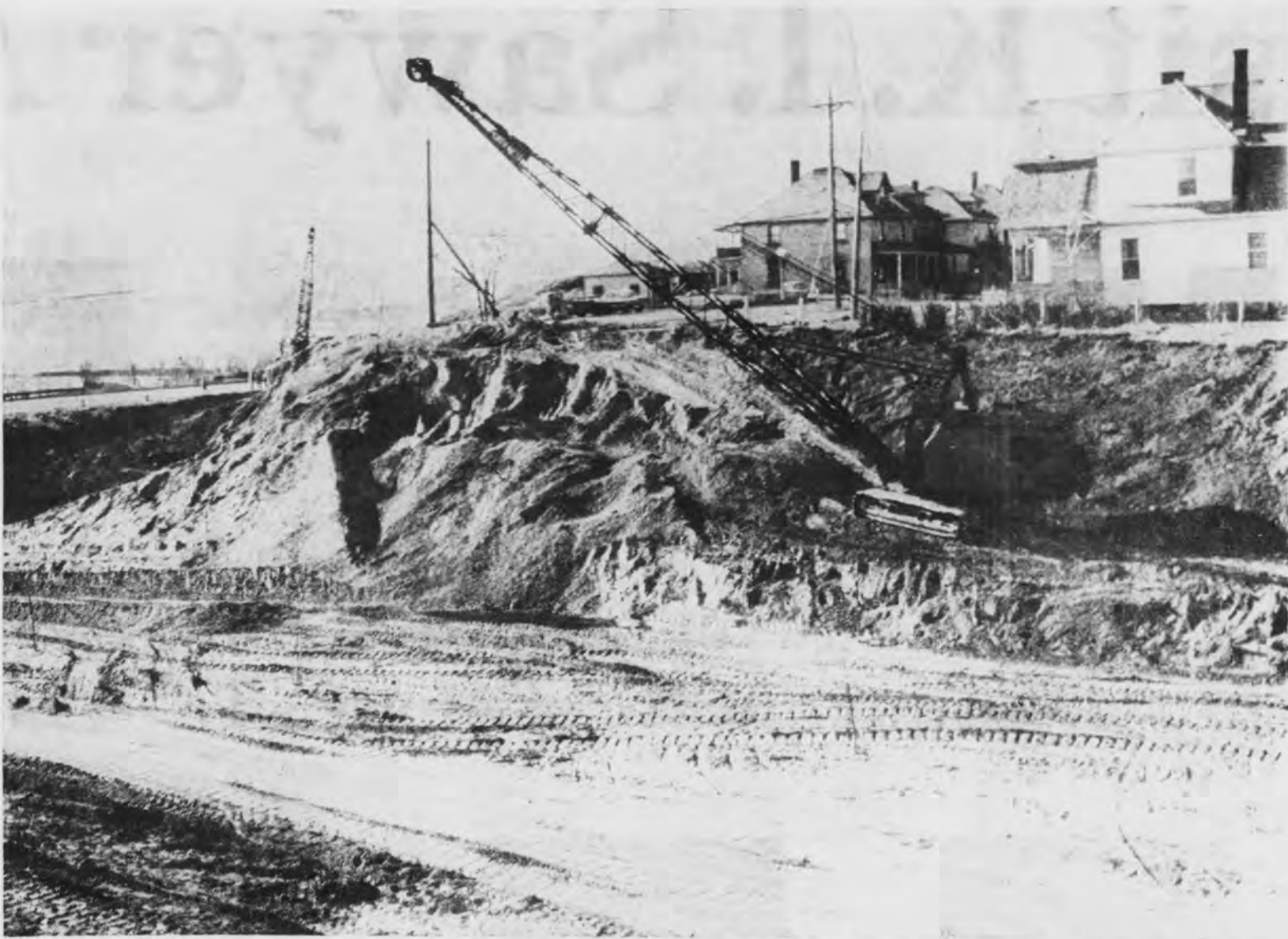
Excavation is proceeding rapidly on the U. S. 41 and M-28 route relocation site for the overpass at Champion St. This scene shows the construction area near S. Front St., U. S. 41 (in background at left). A crane is shown being used to operate a drag line, which has a capacity of two yards. The overpass will provide for the divided four-lane bypass to pass underneath the bridge, which will carry Champion St. (shown near houses) overhead. It is one of two overpasses
