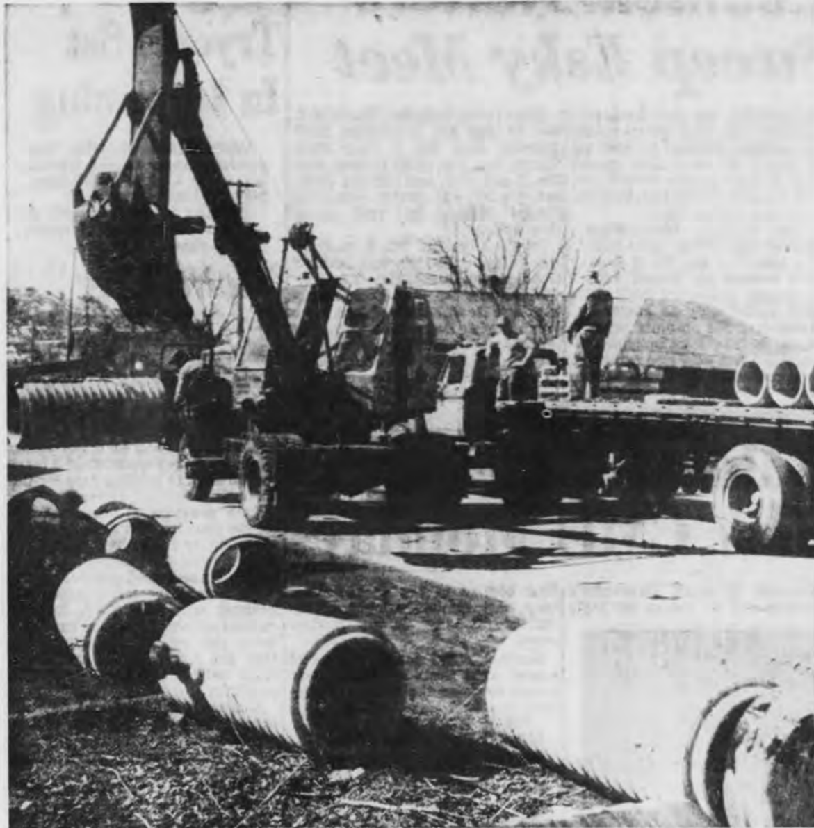
A $236,000 sewer project has been started in Ishpeming by the L. W. Brumm construction firm of Marquette. Eighteen-inch concrete sewer pipes (above) are being unloaded (above) at the corner of Carp and Greenwood Sts. The project is scheduled for completion in February of 1964, but work may be finished in November of this year, according to City Manager Thomas R. McNabb.
