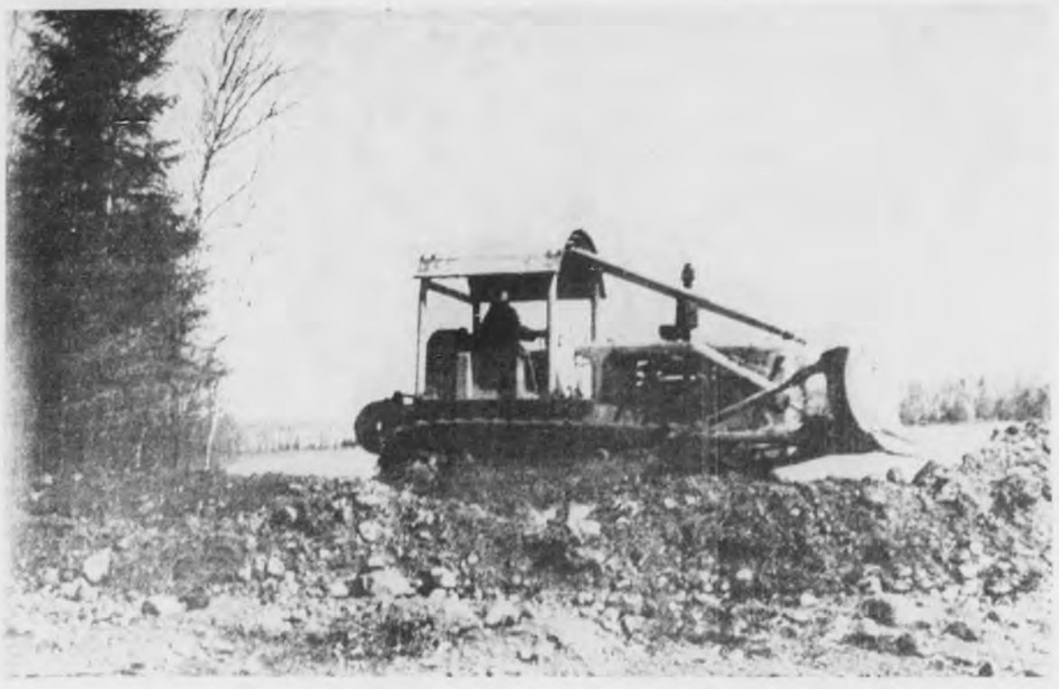
Bulldozer at work on shore of Petticoat Lake. Celotex Corp. crews are constructing access road bed and cutting down high banks and filling low spots. Celotex Corp. crews are constructing access road bed and developing property for cabin sites.
