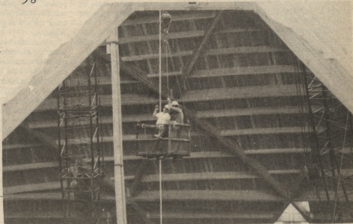
Although behind schedule, the dome should be safely roofed by the time snow begins to fly. Pictured above, two construction workers take the easy way down. (George Hannemann photo)
