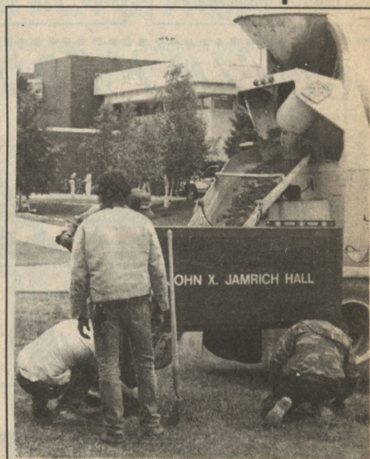
Workers cement the footings of one of the new signs popping up all over campus. (John McNally photo)
