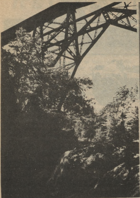
This railroad trestle spanning the Dead River is located approximately five miles west of Marquette, just off of U.S. 41.
