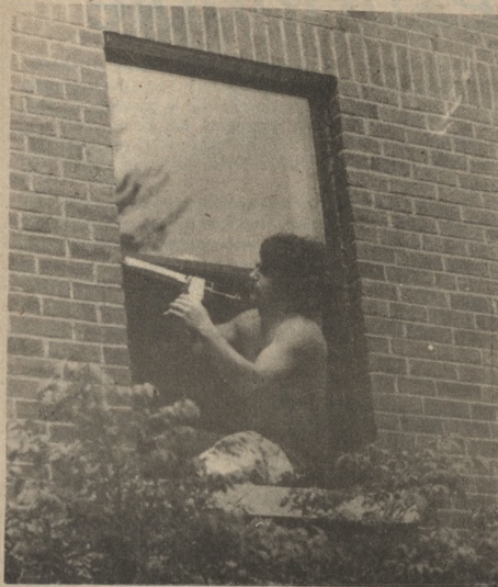
The dormitories around campus got a face lift this summer when 2,440 new windows were installed. The windows are expected to save the University thousands of dollars in energy costs. Students living in the residence halls will be charged a $20 energy fee to help repay the cost of the windows.
