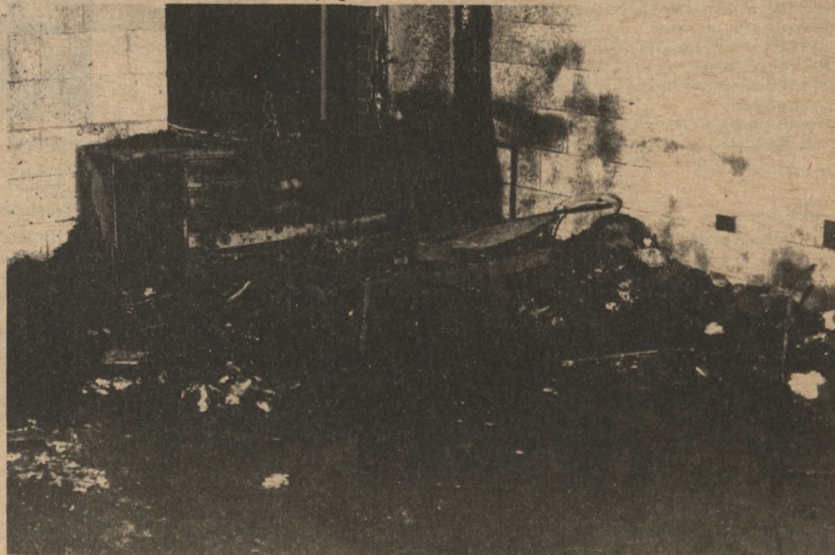
Arson has been cited as the most likely cause in the recent Meyland Hall fires. NMU President John X. Jamrich has said that the damage estimate may run into several thousand dollars. The T.V. room of Meyland's second-floor Oasis House was gutted to the original cement construction said Jamrich.
