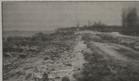
Photo courtesy of City of Marquette Lakeshore Boulevard after a devastating storm in October 2018.
