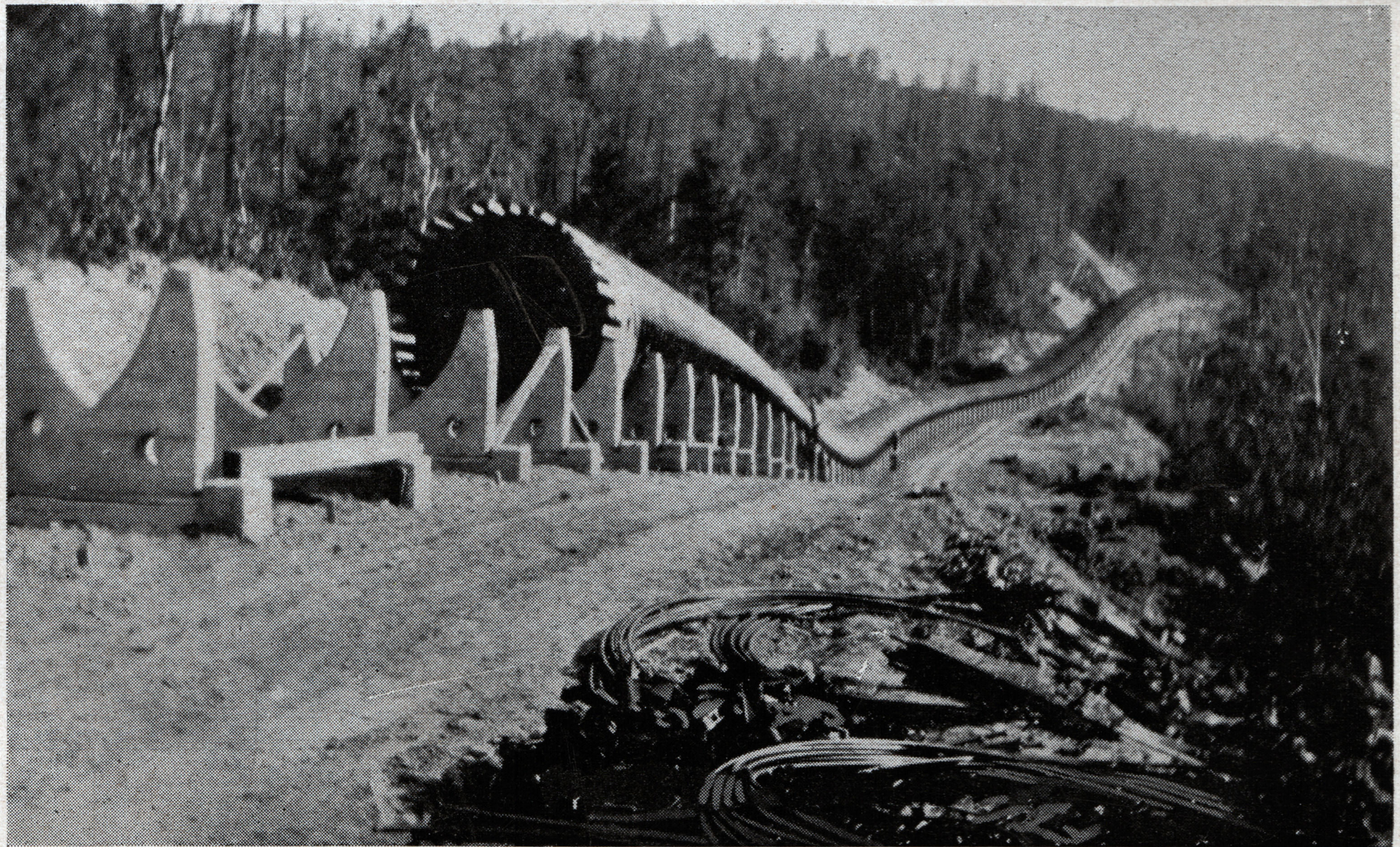
Pipe Line from Dam to Power House at Victoria on Ontonagon River, Line 6,000 feet long, 11 feet diameter
