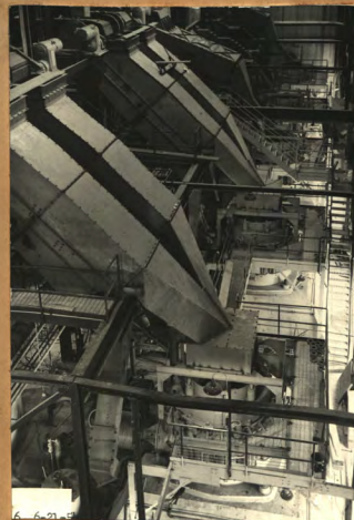
IN THE CRUSHER BUILDING ... ONE STEP IN MILLING THE ORE
