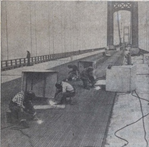
Final touch prior to opening of the Mackinac Bridge (November 1). U. S. Steel's American Bridge Division workmen weld steel bridge flooring sections together. The two inner lanes are of open I-Beam-Lok steel flooring, while outer two lanes are concrete filled. Concrete later was topped with asphalt.
