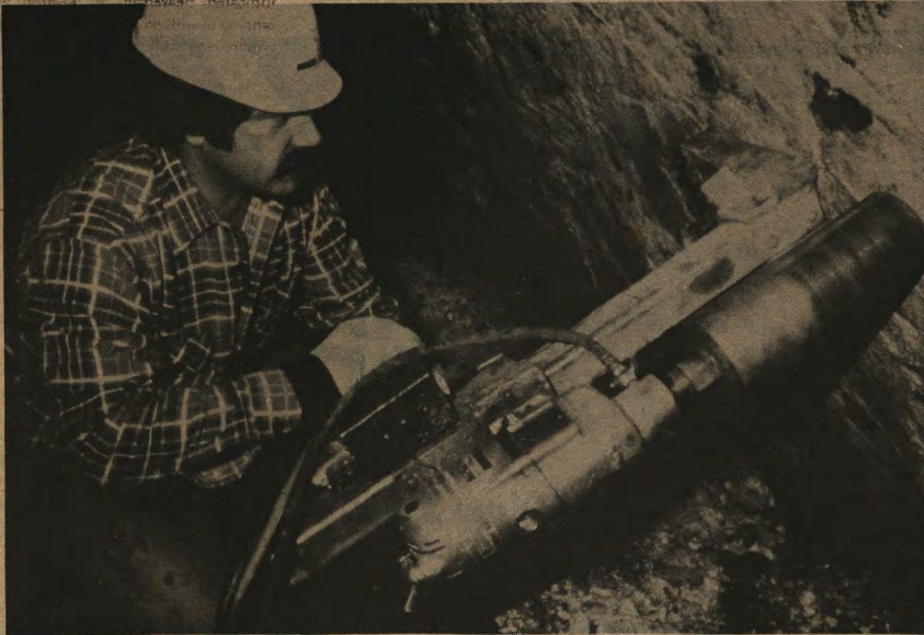
PREPARING FOR MAINTENANCE PROJECT AT VICTORIA DAM, Jim Mishell of Structural Bonding Company, Flint, takes a core sample to determine the internal condition of the dam. The Upper Peninsula Power Company plans to use a specially developed bonding process to repair and reinforce its Victoria hydroelectric facility. (See accompanying story.)
