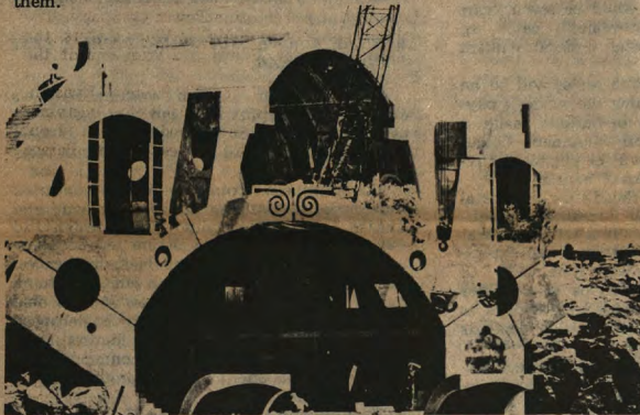
Concrete was placed using silt-casting techniques for apses and vaults of peripheral buildings now under construction at Arcosanti's 860-acre site in Arizona.
