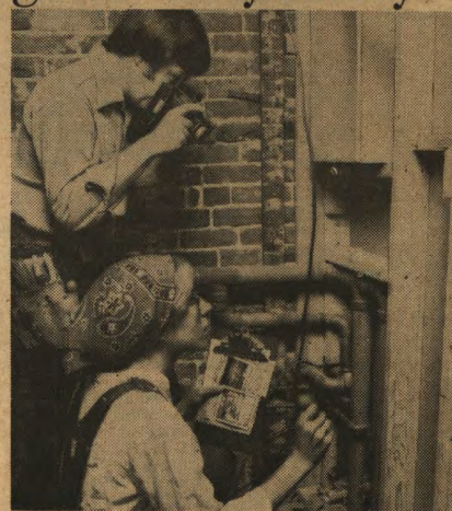
MAKING INSTANT PICTURES of your new walls before they are closed in will give you a valuable record of where all the wires and pipes are inside.
