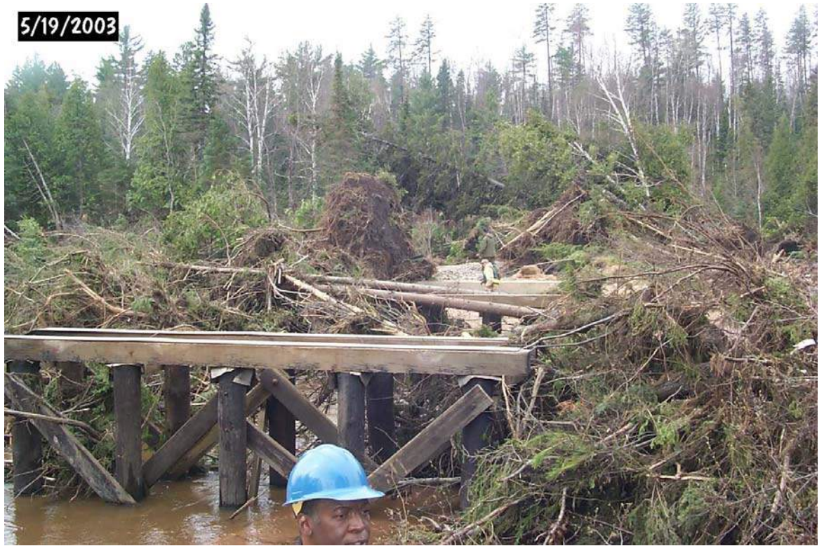
All that is left of the bridge over the Dead River at CR AAO.
