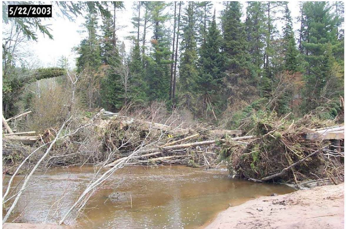
Flood damage at the former bridge over the Dead River at CR AAO.
