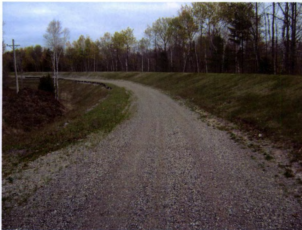
Overall site vegetation between RM-1 and RM-2 (Looking down-stream of penstock flow)
