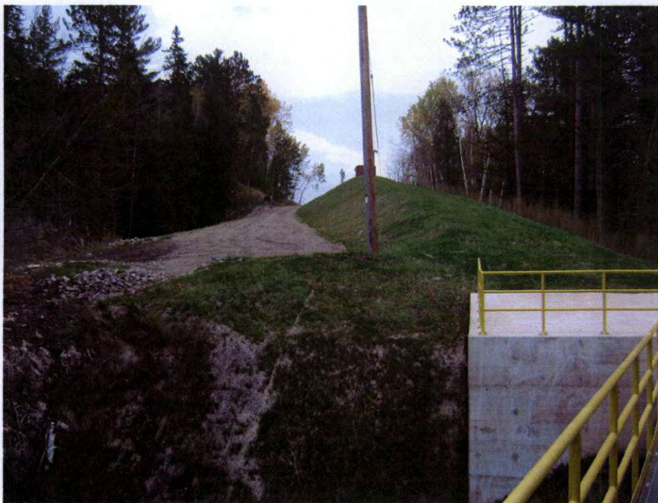
Overall site vegetation between RM-9 and RM-10 (Looking down-stream of penstock flow)
