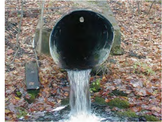
Improperly installed culvert
