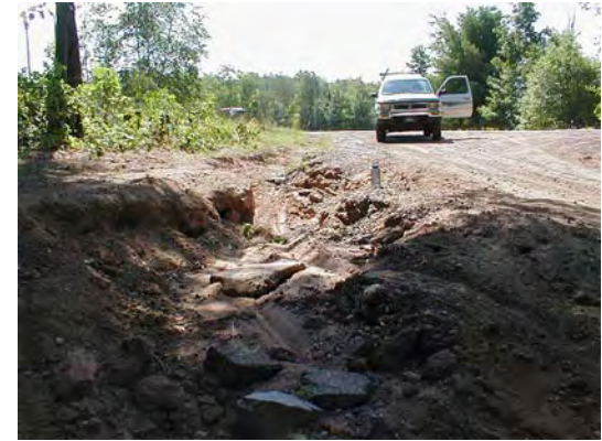
Severe erosion adjacent to Brickyard access road
