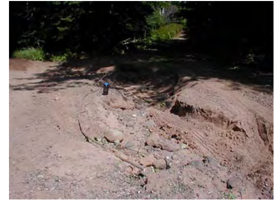
Erosion along the Brickyard Creek access road
