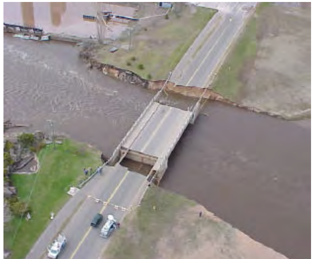
Photo 17. Damaged Lakeshore Blvd. bridge, 5/15/03. Source: Marquette County
