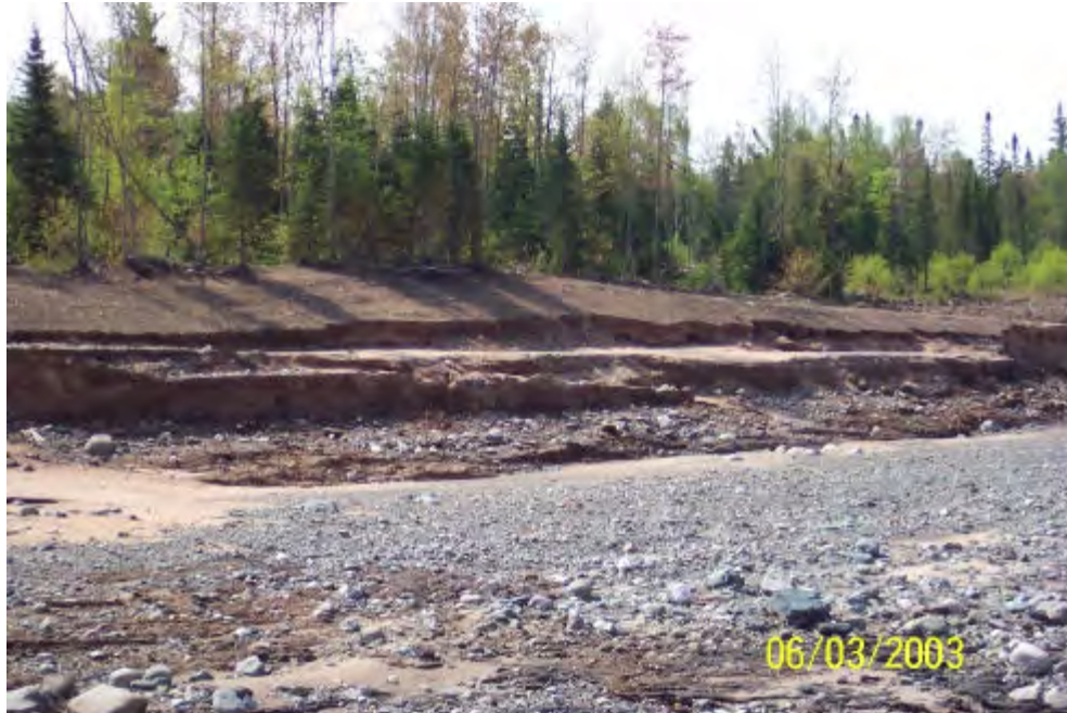
Photo 1. Left bank erosion with remnants of original slope. Upper bench and slope erosion indicates level of initial flow
