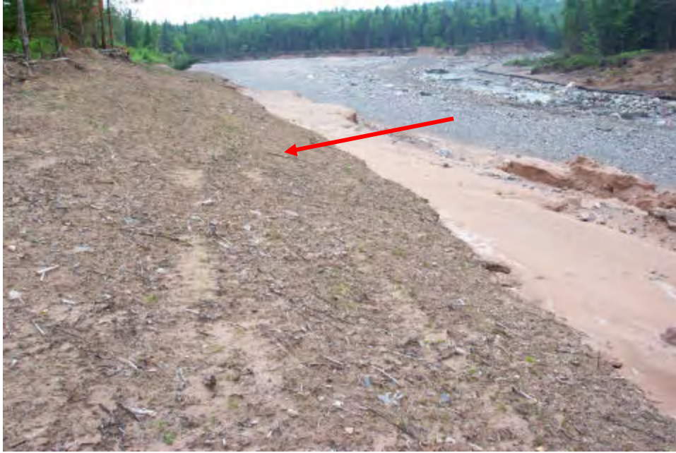
Figure 9 Foreground shows the original ground surface of the fuse plug channel. Flood erosion occurred to the right of the line marked by the arrow. Note the coarse-grained cobble and boulder deposition along the channel centerline. View is on left channel downstream of former fuse plug.
