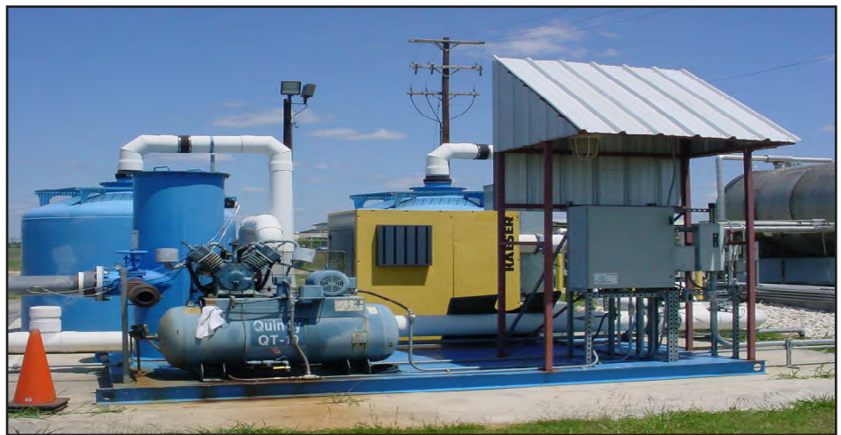
A soil vapor extraction system used at the former Kelly AFB.
