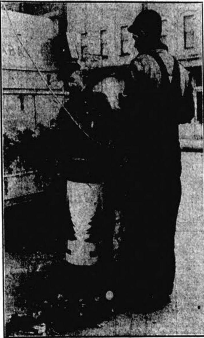
City employes yesterday installed Christmas lighting decorations with evergreen streamers at the intersections of Ludington street. Lights are contained in the cylindrical container shown above.
