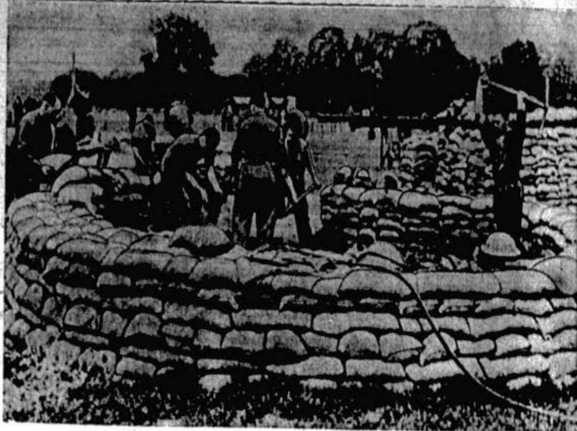
In an attempt to surround London with a ring of steel and prevent "death from the skies," British troops rushed the building of sandbag emplacements (as in park above) and erected anti-aircraft guns about the city. (NEA Cablephoto)
