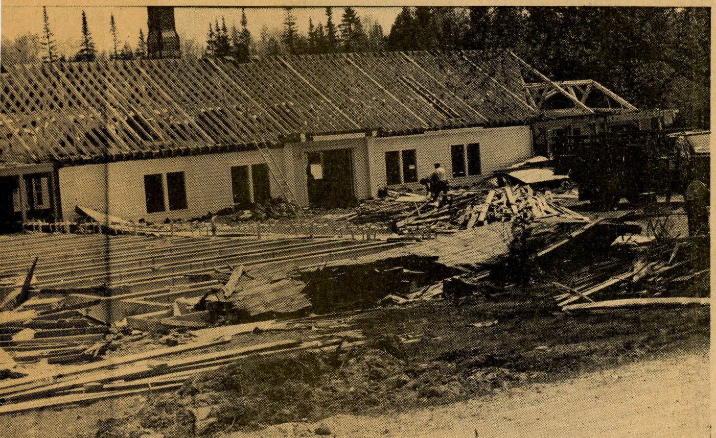
DEMOLITION WORK on the upper unit of the Thompson Fish Hatchery is proceeding on schedule. Much of the material from the building will be utilized in the construction of the new hatchery building. (Tribune photo)
