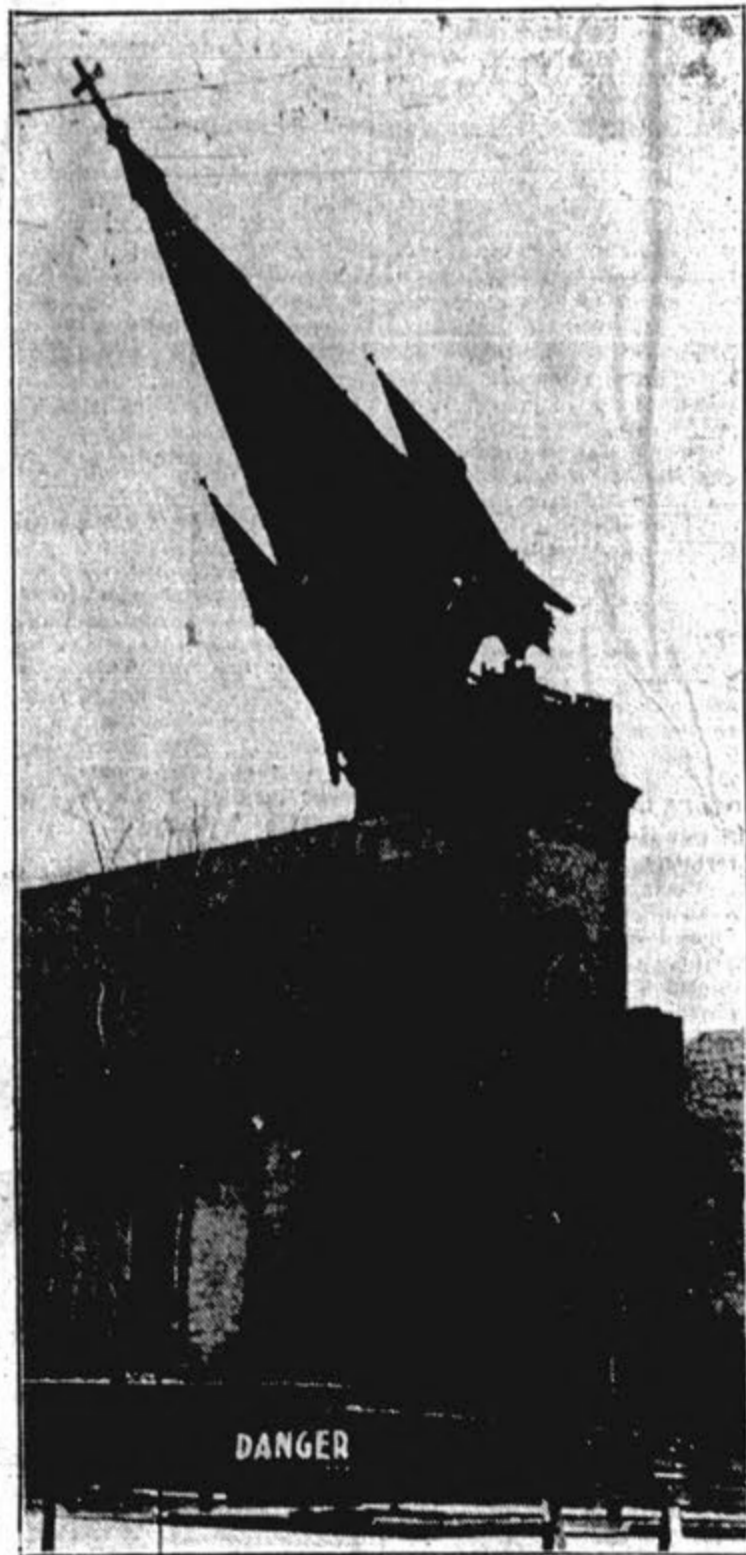
CAUGHT IN MID-AIR by the Daily Press camera was the steeple of St. Joseph's Catholic church, which toppled to the ground the morning of May 6 as workmen demolished the old structure to make way for the new building now under construction on the same site.
