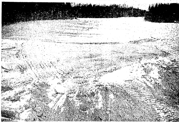
MAIN ROUTE---The new pipeline stretching across the countryside provides a ready-made route for snowmobiles, as these tracks in the snow can prove.
